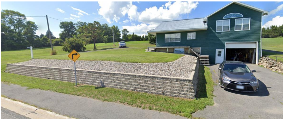
Figure 1: Retaining Wall Subject to Encroachment
